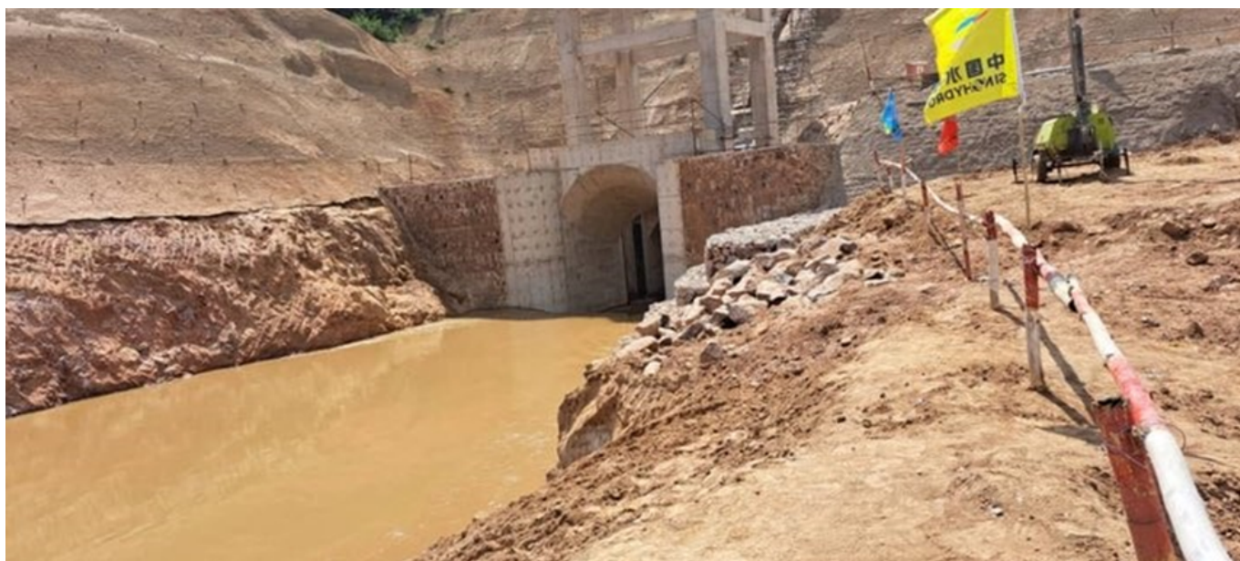
Nyabarongo II Hydroelectric Power Station, with installed generating capacity of 43.5 megawatts.
